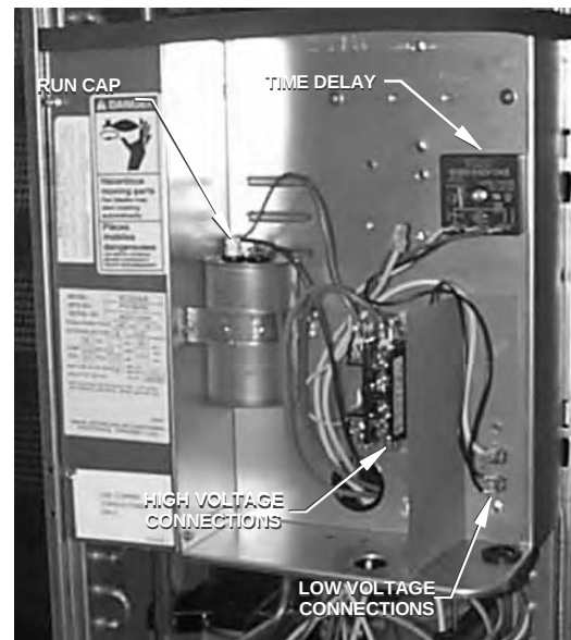
Figure 7 Unit Control Panel
